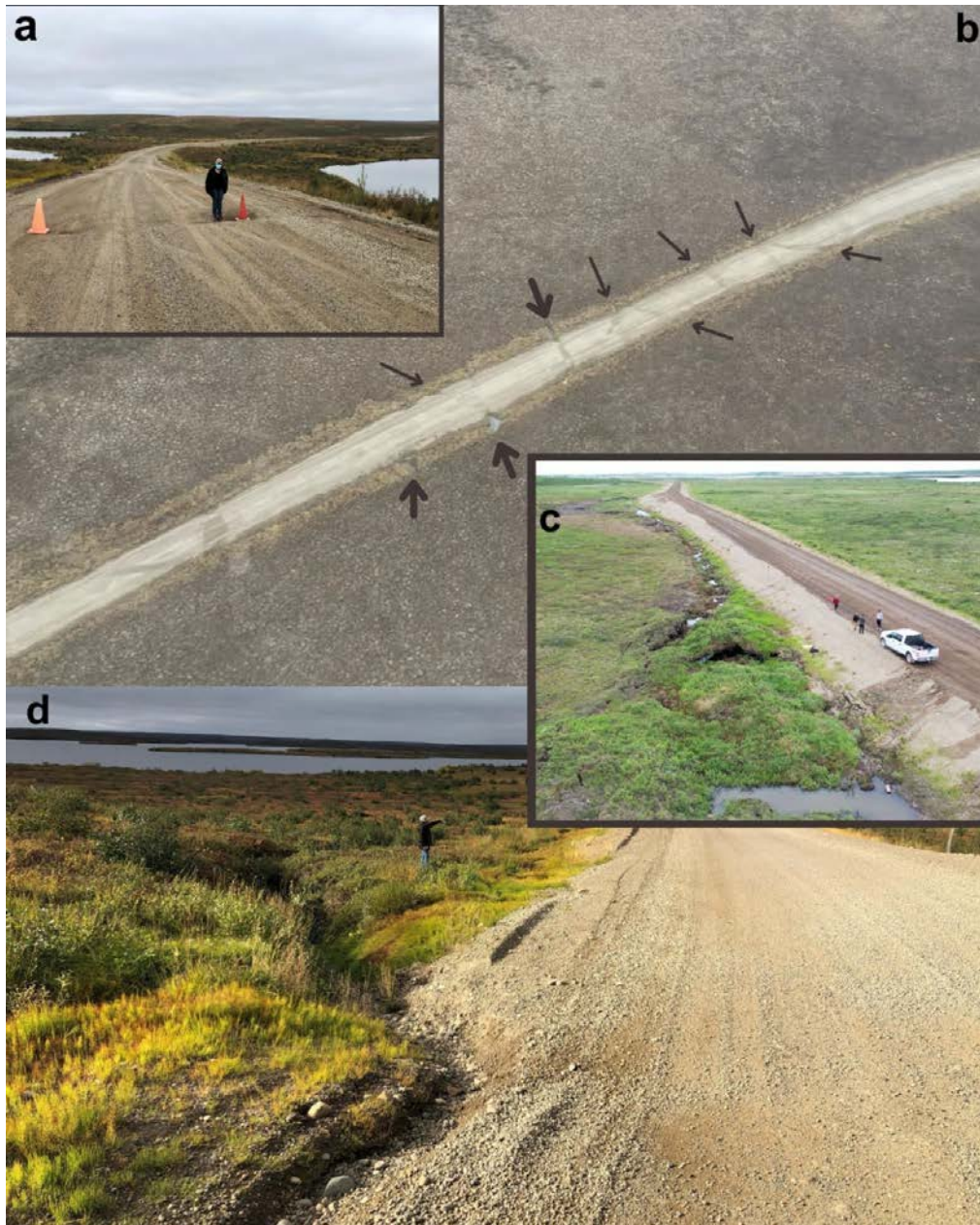
↑ Disturbances along the ITH. (a) "A depression caused by ice wedge thaw and surface subsidence at km 100." Photo credit: GNWT – Jurjen Van der Sluijs, August 2022. (b) "An aerial view of ice-wedge degradation beneath the highway embankment at km 46, with the thin arrows indicating degraded troughs and thick arrows indicating degraded troughs with ponds at the embankment edge." Photo credit: Aurora College – Celtie Ferguson, September 2023. (c) "Ponding, embankment sloughing, degrading ice wedges, and a heaved mat of organic materials from a large icing and frost blister that developed in the winter 2020/21 at km 106." Photo credit: Aurora College – Celtie Ferguson, June 2021. (d) "Erosion of the road embankment and degraded ice wedges beside the road at km 84." Photo credit: GNWT – Jurjen Van der Sluijs, August 2022.
