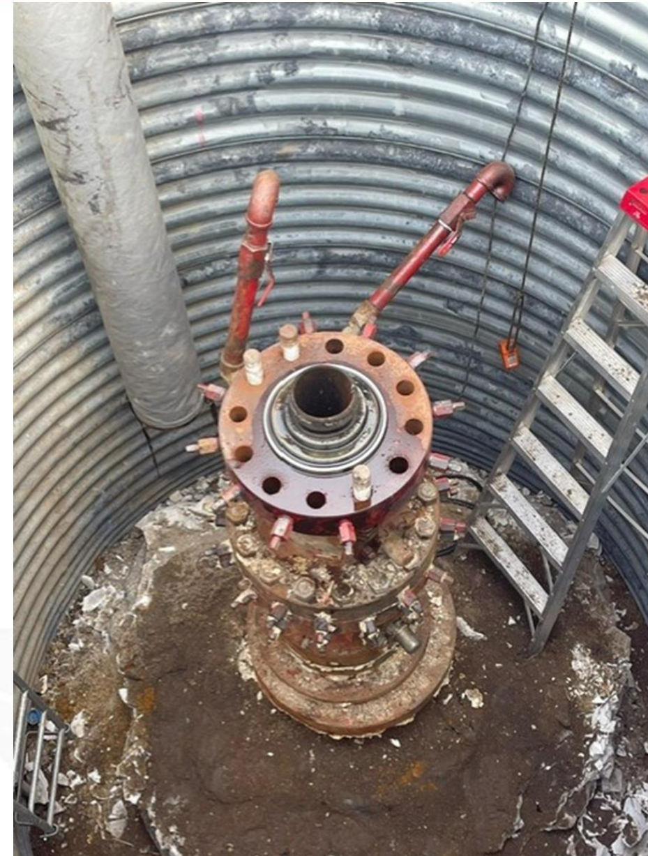
Casing Stump Without Wellhead
